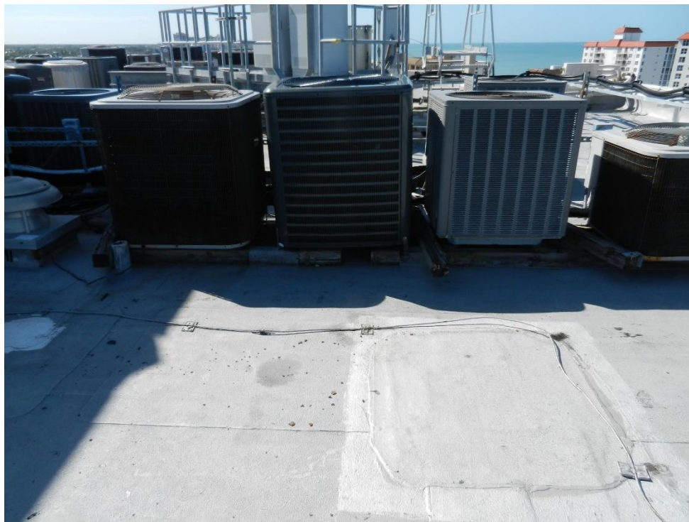
Deteriorating HVAC Support
