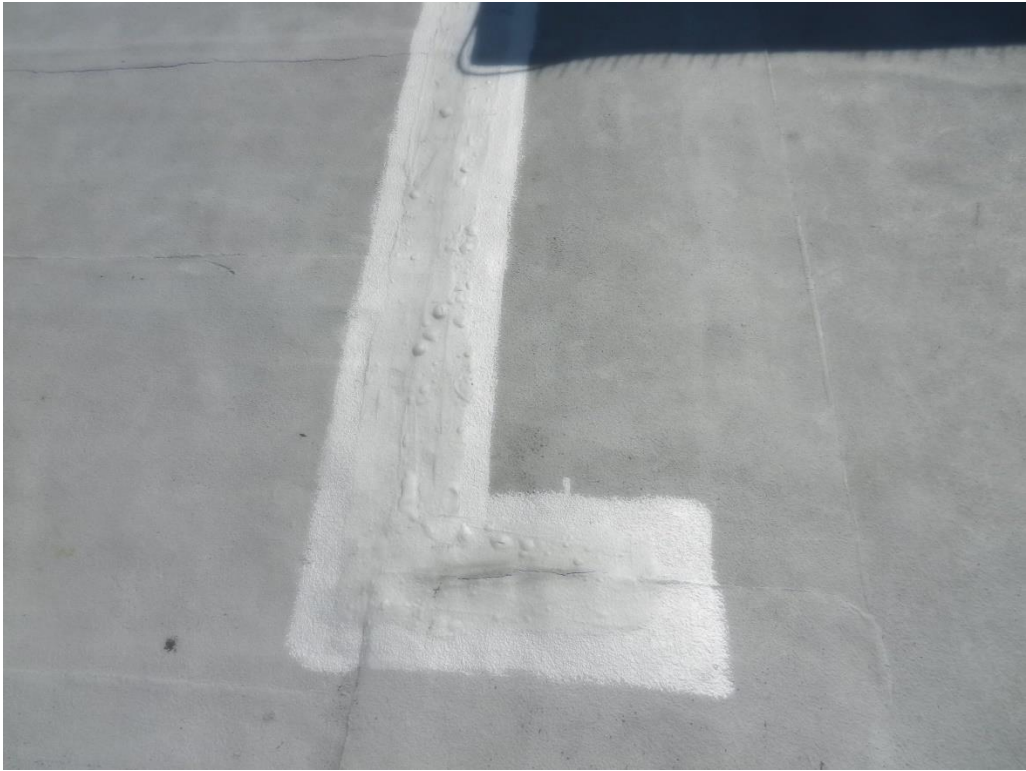
Potential Roofing Failures
