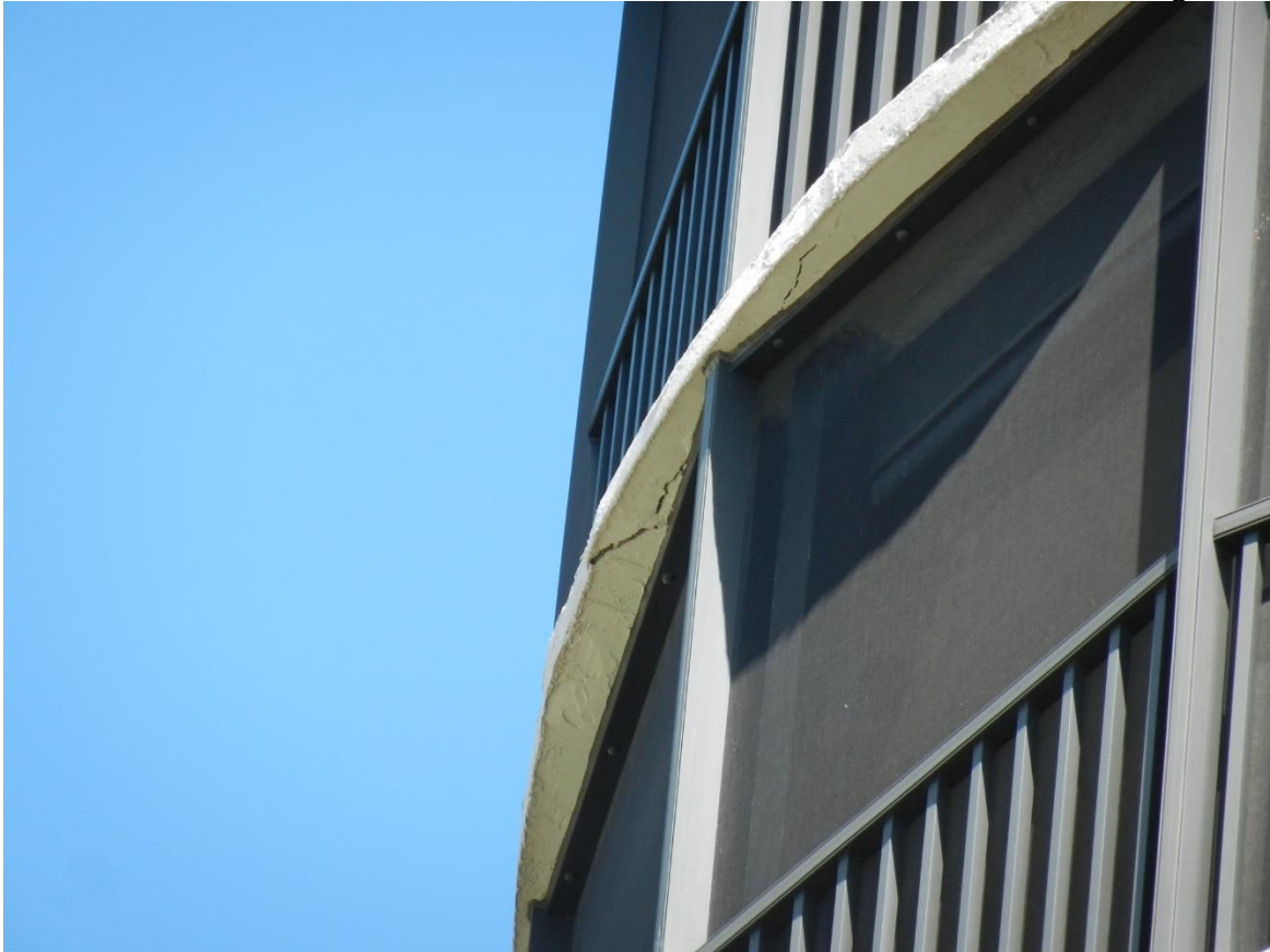
Lanai Deck Crack at Unit 903
