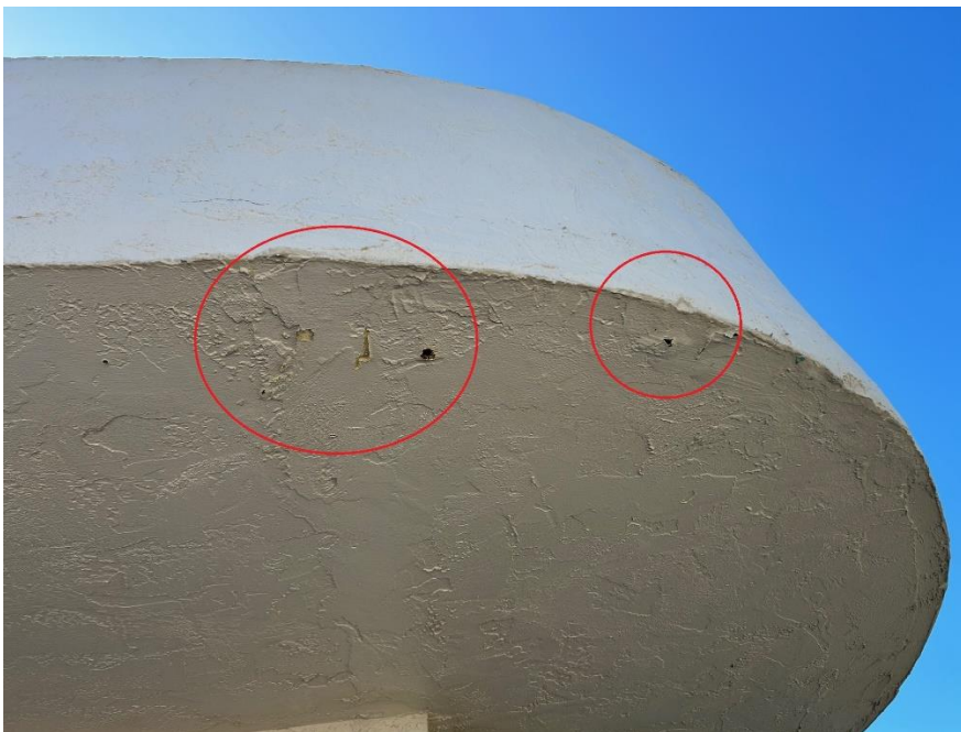
Deteriorating Concrete and Rebar North East Corner of the Roof Deck
